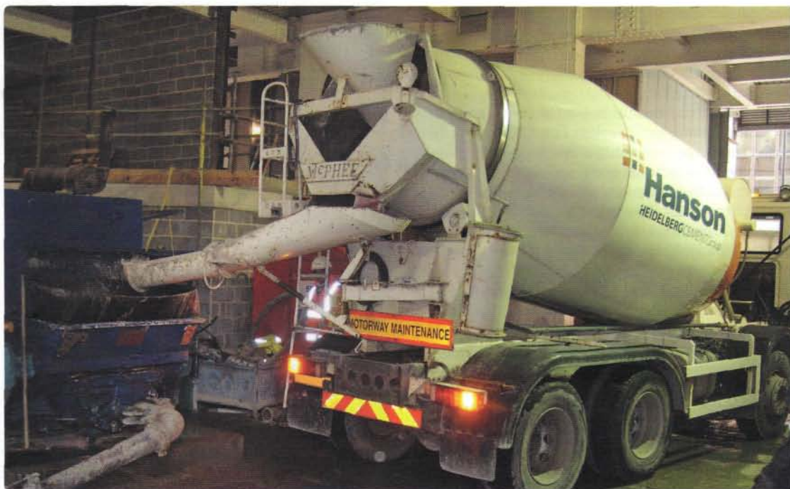
A Hanson truck mixer at Heron Tower. The operator awaits site instruction to discharge lightweight concrete.
