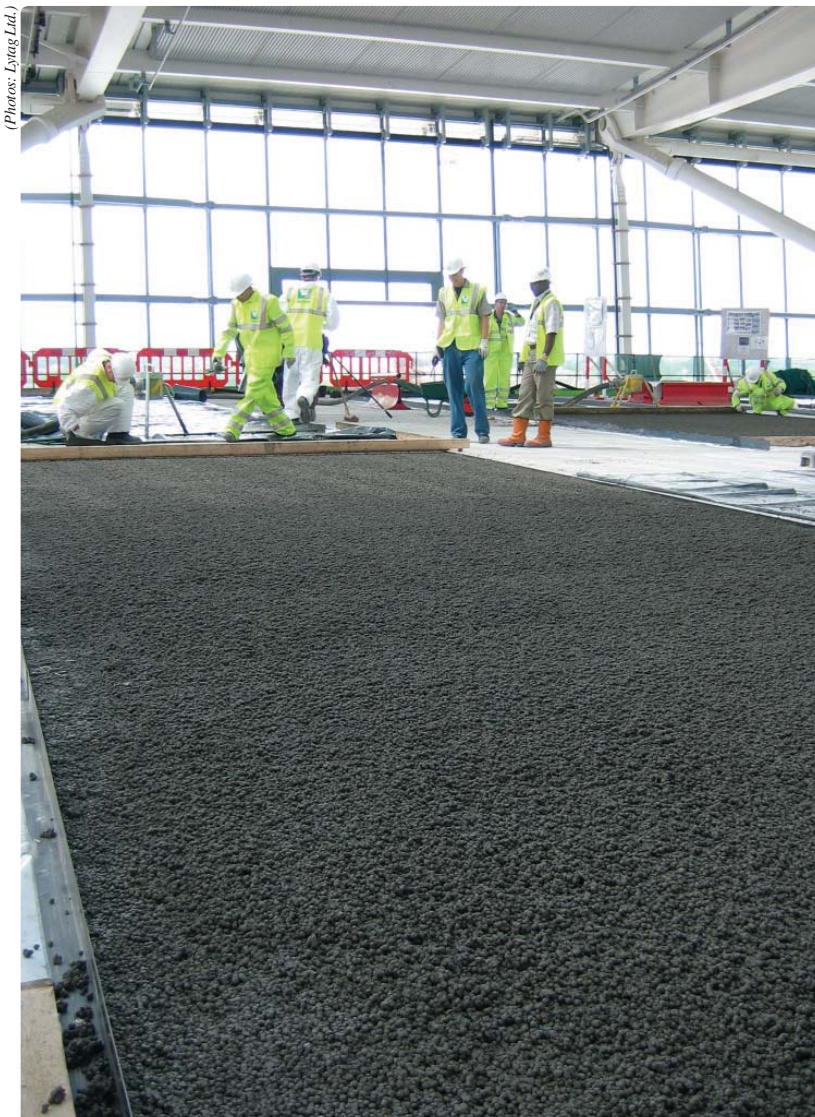
Figures 1 below and 2 opposite: The use of Lytag in the construction of Heathrow T5.
