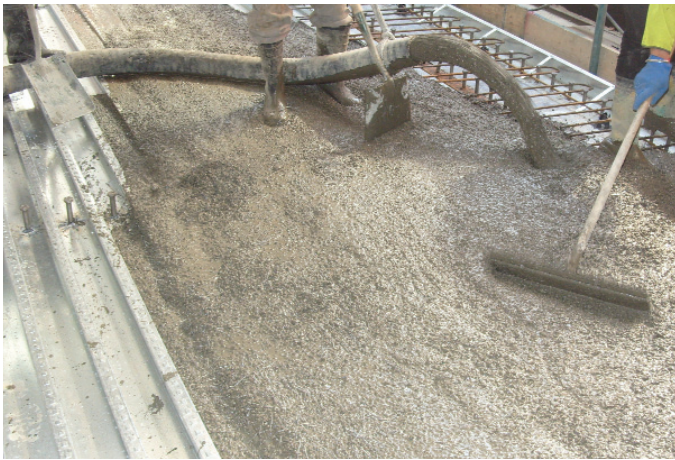
10 Old Bailey – lightweight aggregate concrete used with Strux® synthetic fibres to reduce overall loading on the structure
