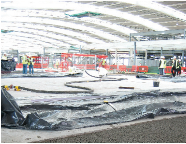
T5 – lightweight aggregate no fines screed used on the main floor areas to reduce loading
